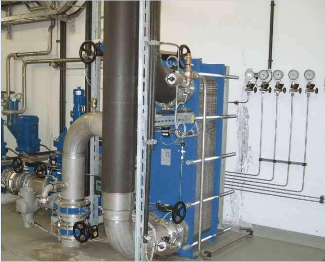
Hydraulic oil cooling in power plant.
