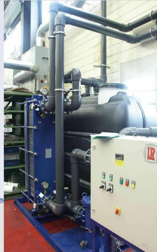
Cooling of lubricating oil for extruding presses.
